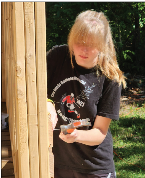
A Cabin Crew camper nails siding onto the new cabin at Camp Farnsworth. (Courtesy photo)
