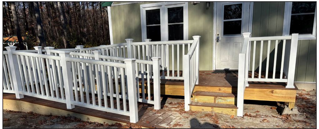
The new ADA-compliant ramp built at Ranger's Roost at Camp Seawood. (GSGWM photo)
